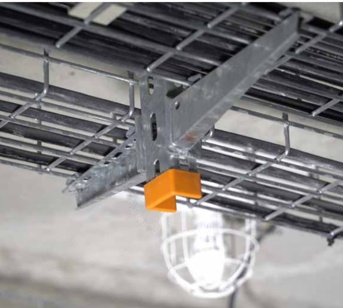
Magic mesh cable tray fitted to a ceiling with a suspended support and brackets on either side
