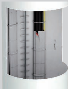
Bandaged rising section in the tower of a wind power plant.
