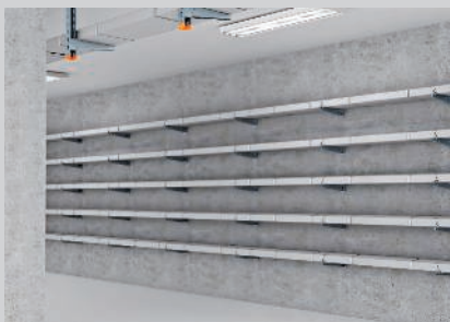
Cable tunnel with bandages in power stations.
